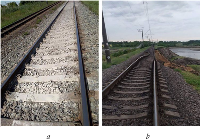
Figure 1. Defective places of the roadbed (a) a section of railway track with spills, (b) loss of stability of the slope of the roadbed due to soil compaction
